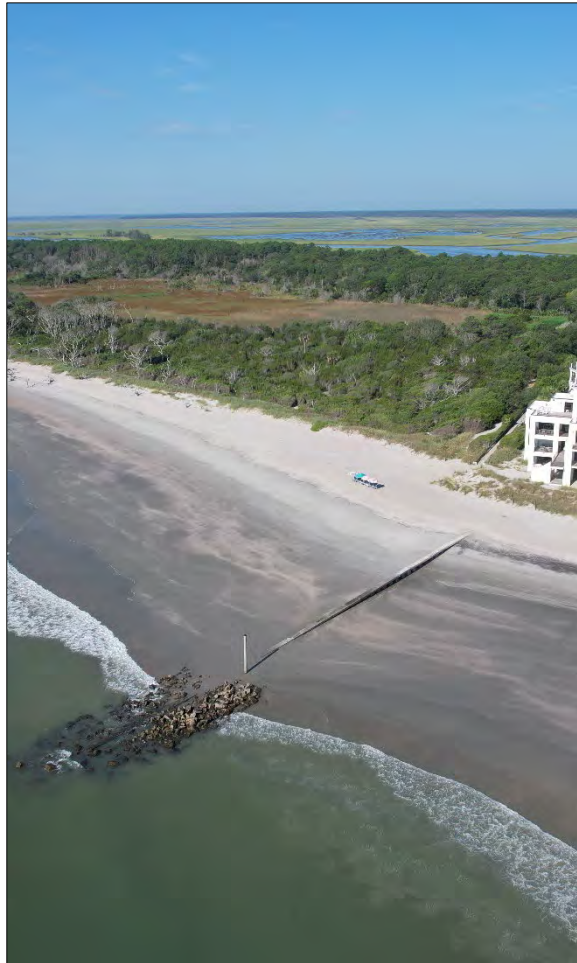
FIGURE 4.17. Groin #3 oblique aerial, July 2025. Much of the structure exposed above MLW.
